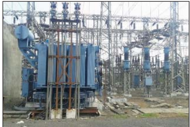
Transmission line at Margarwada, Daman
