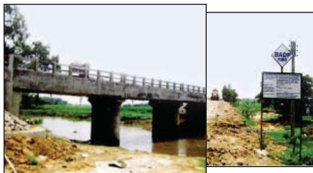
Construction of Bridge over Akhiradanga Khari (Phase-II), Tapan Block District: Dakshin Dinajpur (West Bengal) under BADP
