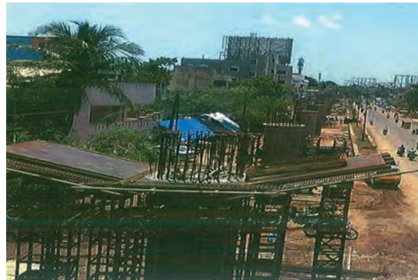
Road Over Bridge across LC 43A on 100 Feet Road, Puducherry - Work in progress
