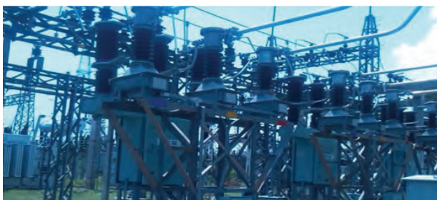
A view of the renovation and modernisation works carried out at Villianur 110/22KV Sub-station.
