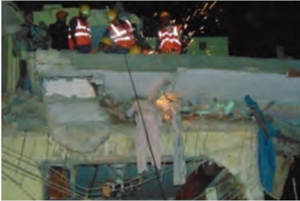
NDRF rescuers during building collapse rescue operation at Khyala, Delhi
