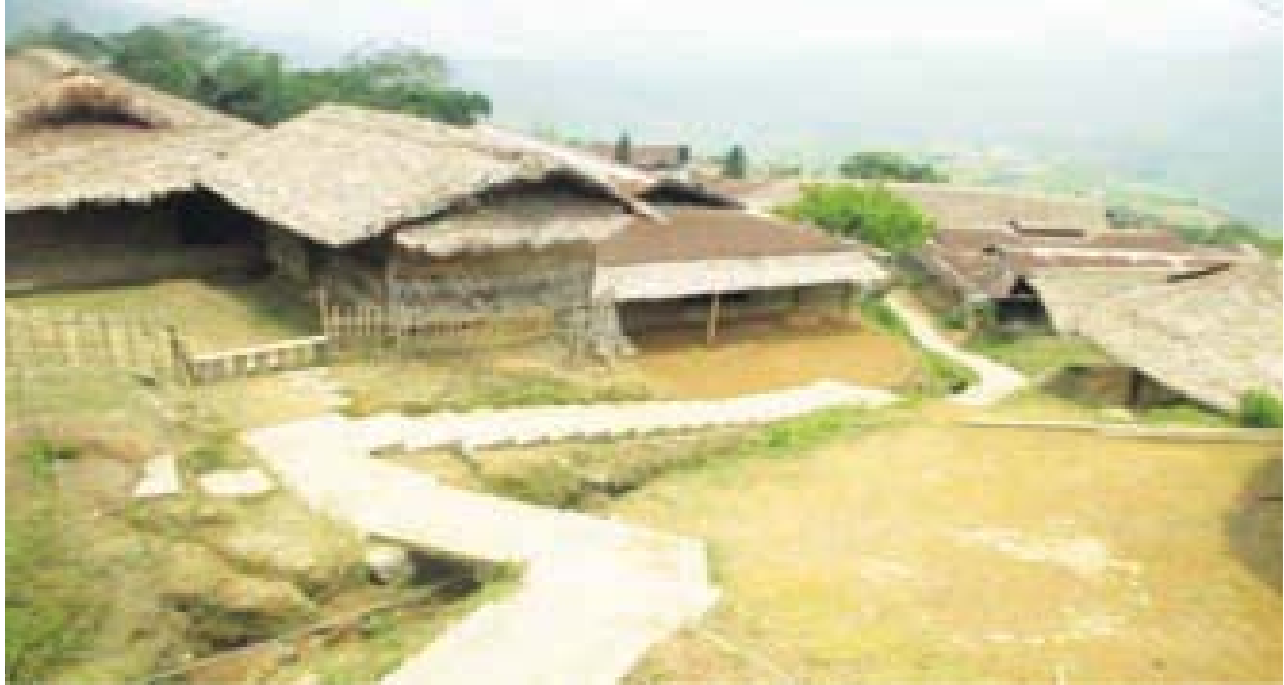
Construction of Footstep at Chingkao Chingha village, (District: Mon) Nagaland under BADP, SCA: 2014-15
