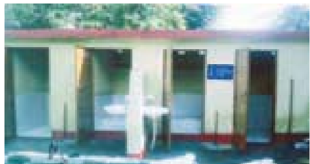
Construction of Public Toilet at Kapra Thaur village (District: Pithoragarh) Uttarakhand under BADP, SCA: 2014-15
