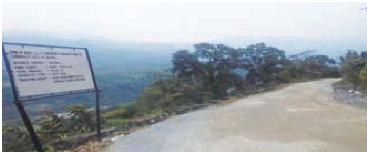
Construction of CC Pavement from BRTF Road to Community Hall at Gossing village, District Upper Siang (Arunachal Pradesh) under BADP, SCA:2015-16)
