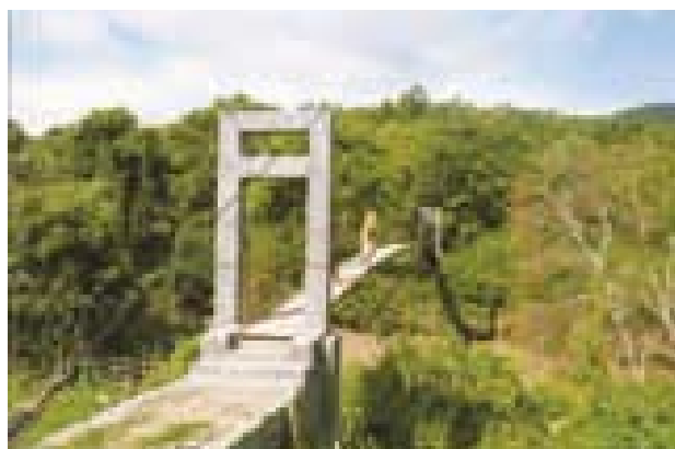
Construction of Suspension Bridge over Tuival river at L. Kanan Village (District: Churuchandpur) Manipur under BADP, SCA: 2014-15
