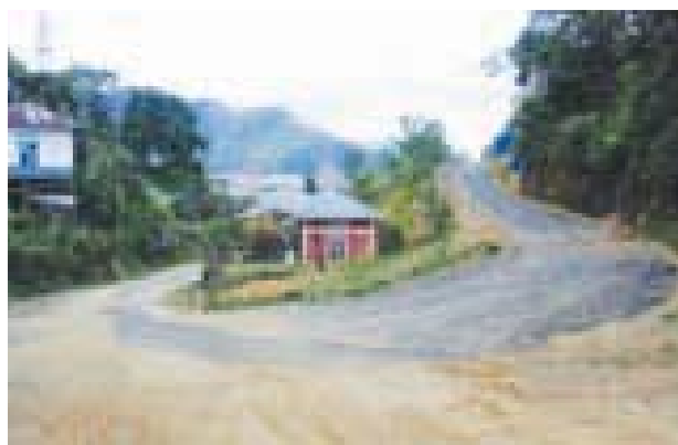
Blacktopping of Internal Road from main Road to Sunday School Hall near 14 th AP Post Khawbung (District: Champhai) Mizoram under BADP, SCA:- 2014-15
