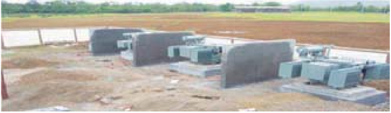
3 MV Solar Power Plant at Velugam
