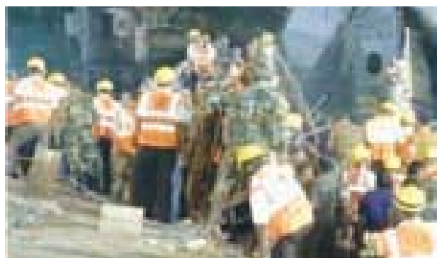
NDRF rescuers during under construction Vivekanand Flyover in Kolkata (West Bengal) collapsed
