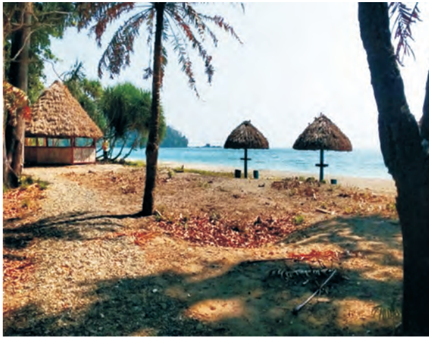
Beach development works and construction of eco-friendly hut at Ramnagar beach under Mahatma Gandhi NREGA
