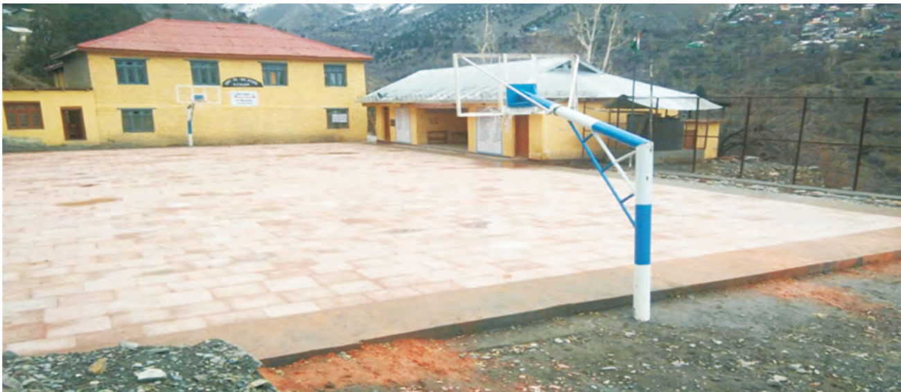
Construction of Play field/Basket Ball Court at Government Sr. Sec. School, Kanam, District Kinnaur (Himachal Pradesh) under BADP, SCA: 2016-17
