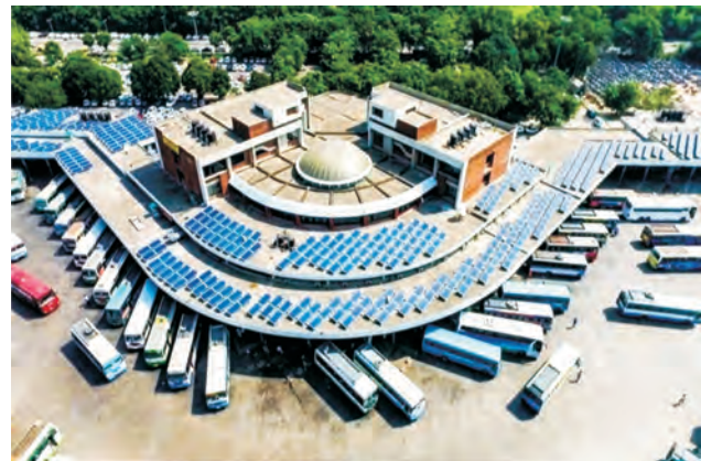
200 KwP Solar Power Plant installed at ISBT Sector 43, Chandigarh
