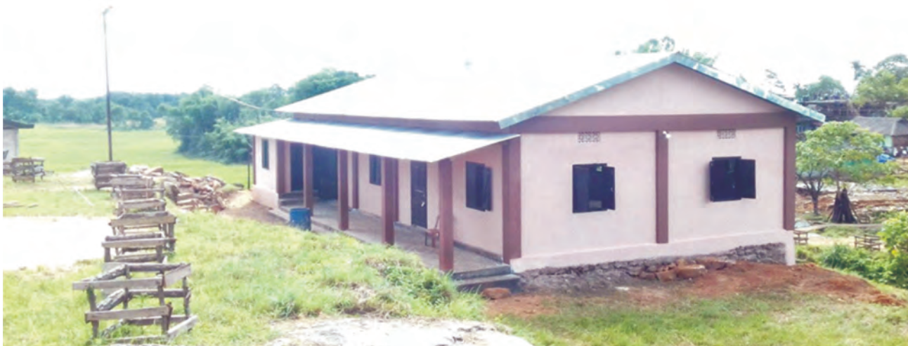
Construction of Community Hall at Umlatdoh, District East Jaintia Hills (Meghalaya) under BADP, SCA: 2016-17
