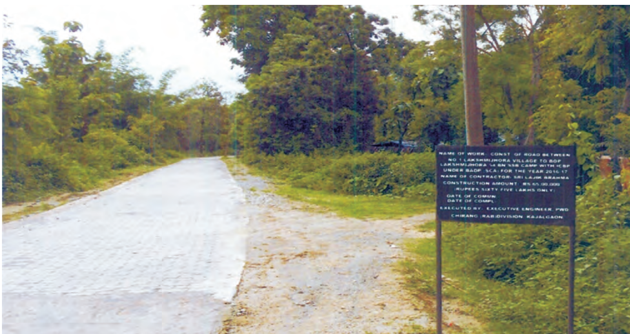
Construction of road between No.1 Lakshmijhora Village to BOP Lakshmijhora 54 Bn. SSB, in District Chirang (Assam) SCA: 2016-17
