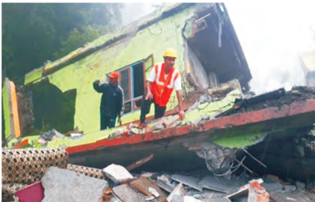
NDRF rescuers saved 03 precious lives who got trapped under the debris of collapsed buildings due to land slide at Pakyong, East Sikkim.
