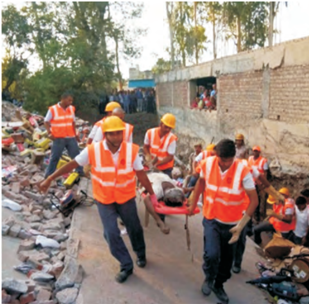
NDRF Rescuers saved 02 victims alive who got trapped under the Debris of Collapsed Building at Jasur, Nurpur ( Himachal Pradesh) on 17.06.2017
