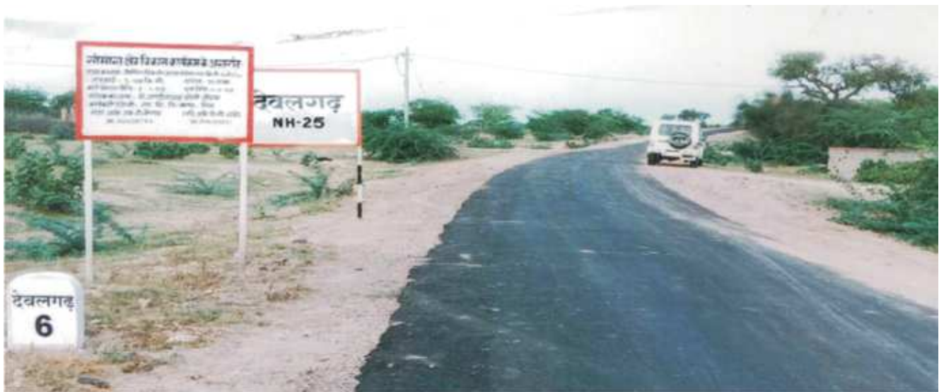
Construction of missing Link Road in Rajasthan from Utarba to Devalgarh N.H 25 Date of Completion: 02.03.2019
